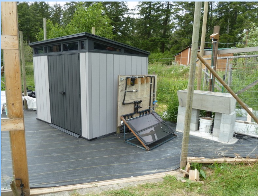
Solar panels and watering control system
