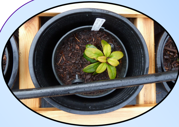
Irrigation drip line
